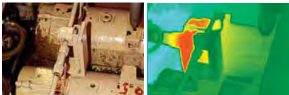
Motor: Bearing Problem.
