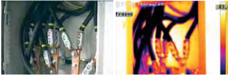
This thermal image looks quite odd, if you don't know the circumstances under which it was taken. The cables are not loaded at all. They are located in a warm room and the non-oxidized metal surfaces reflect the warm ambient temperature.
