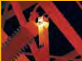
Incorrectly secured connection
