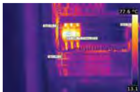
The fuses that show up in the thermal image are overloaded and need to be replaced.
