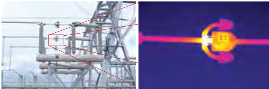
Thermal imaging cameras allow you to inspect high voltage installations from a safe distance, increasing worker safety.
