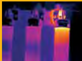
Internal fuse damage
