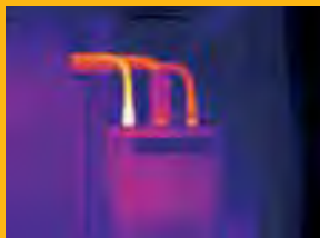
Poor connection and internal damage
