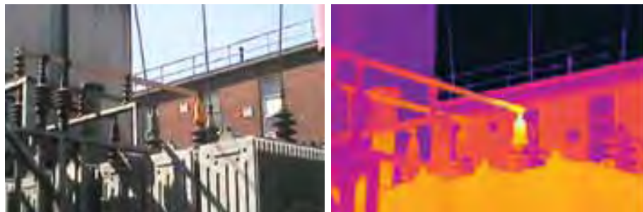
A wide view of a substation can quickly show areas where unwanted high resistance connections exist. No other predictive maintenance technology is as effective for electrical inspections as thermal imaging.
